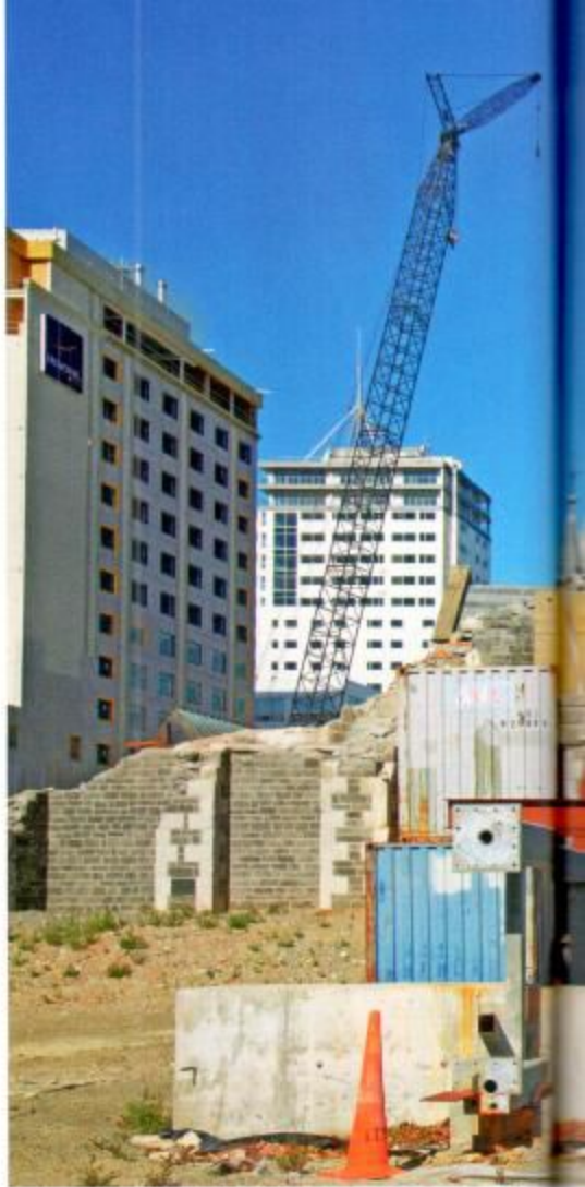
The view (far right) from atop the Ibis Hotel, captured in December 2012, shows the edge of the red zone, where construction is underway. Christchurch's cathedral (above), a city icon, is earmarked for demolition but a battle continues for its survival. Christchurch Mayor Bob Parker (right, at right), and North Island-based politician Phil Goff pause during a minute's silence for the 2011 quake victims.
